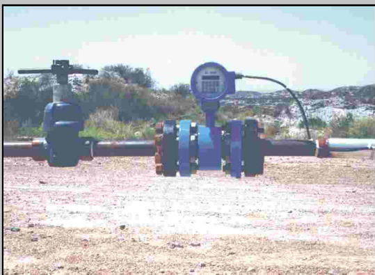
Equipment mounted at an oil field in Tupungato, Province of Mendoza
